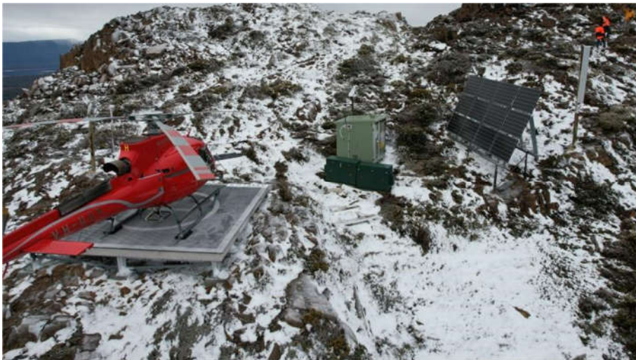
FIGURE 4 INTERNAL VIEW OF SITE SHOWING HELIPAD AND TMRN SHELTER AND BATTERY BANKS AND SOLAR ARRAY
