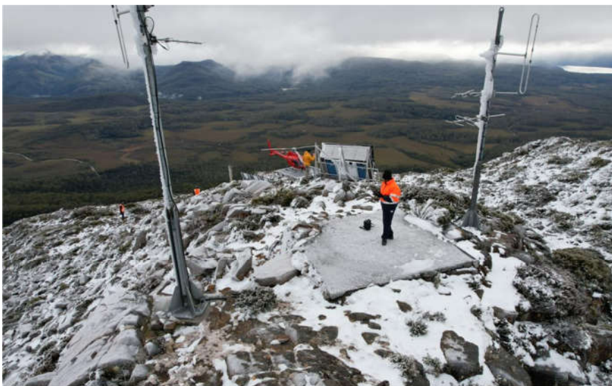
FIGURE 6 INTERNAL VIEW OF SITE SHOWING VACANT BITUMEN PAD WHERE PROPOSED TASGRN MAST AND OMNI ANTENNA WILL BE LOCATED AND 5M FOLDABLE MONOPOLES
