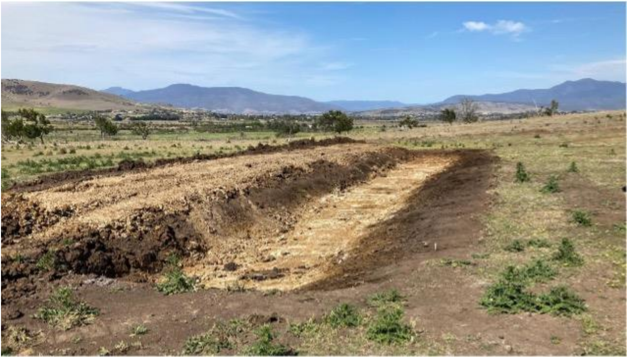
Figure 7-1: Biosolid stockpiling bund. Trucks unload on the right-hand side and the excavator loads the spreader on the left. A small berm on the loading site is added (not shown in picture) to prevent surface water entering and to provide a stop for the back wheels of the trucks (photo provided by Spectran).
