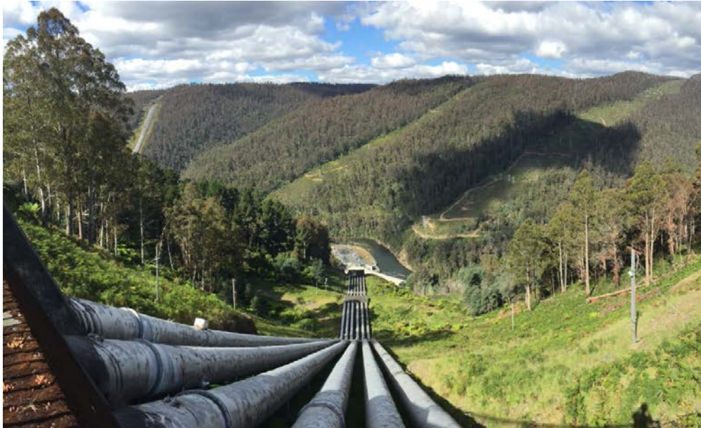
Photograph 1 Penstocks at Tarraleah provide high scenic interest (Source: Creative Commons 29 )
