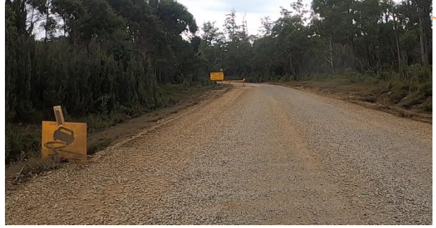
Figure 9: Butlers Gorge Road - dirty signs and missing taper (-42.297, 146.382)
