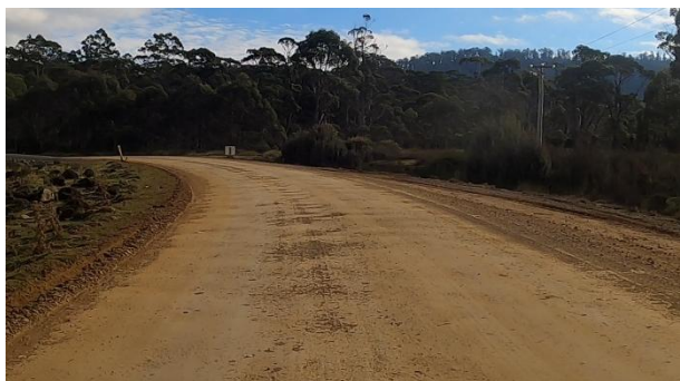
Figure 6: Butlers Gorge Road - evidence of minor corrugations (-42.266, 146.291)
