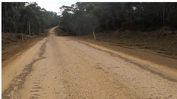
Figure 4: Butlers Gorge Road - evidence of longitudinal scouring (-42.282, 146.400)
