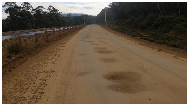
Figure 5: Butlers Gorge Road - evidence of minor potholes (-42.267, 146.316)
