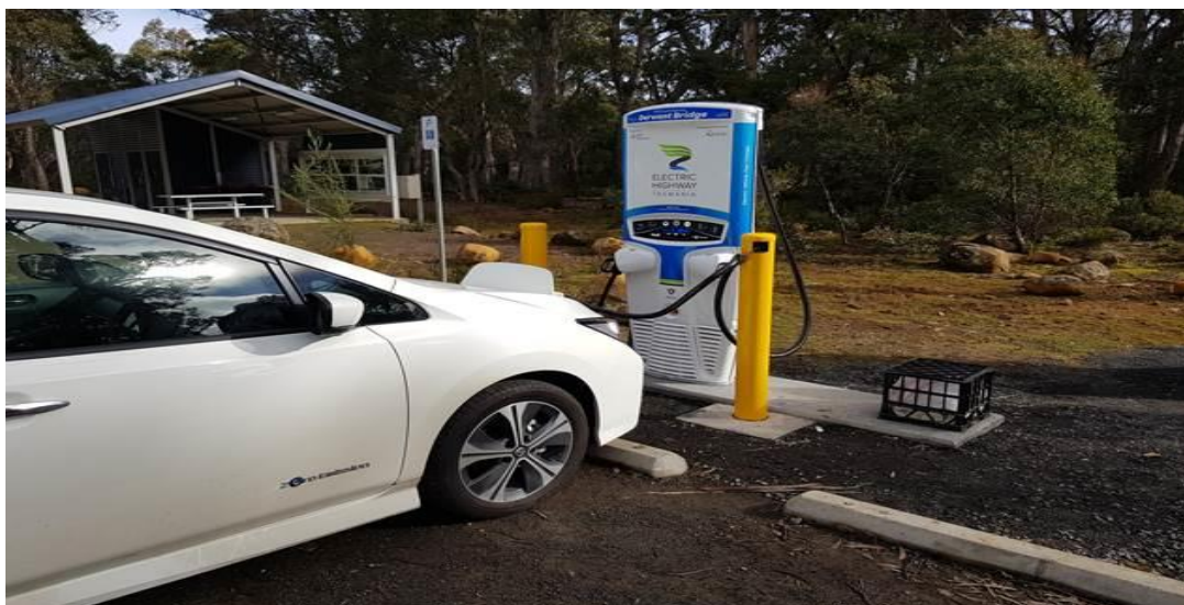
Electric Fast Car Charger at Derwent Bridge
