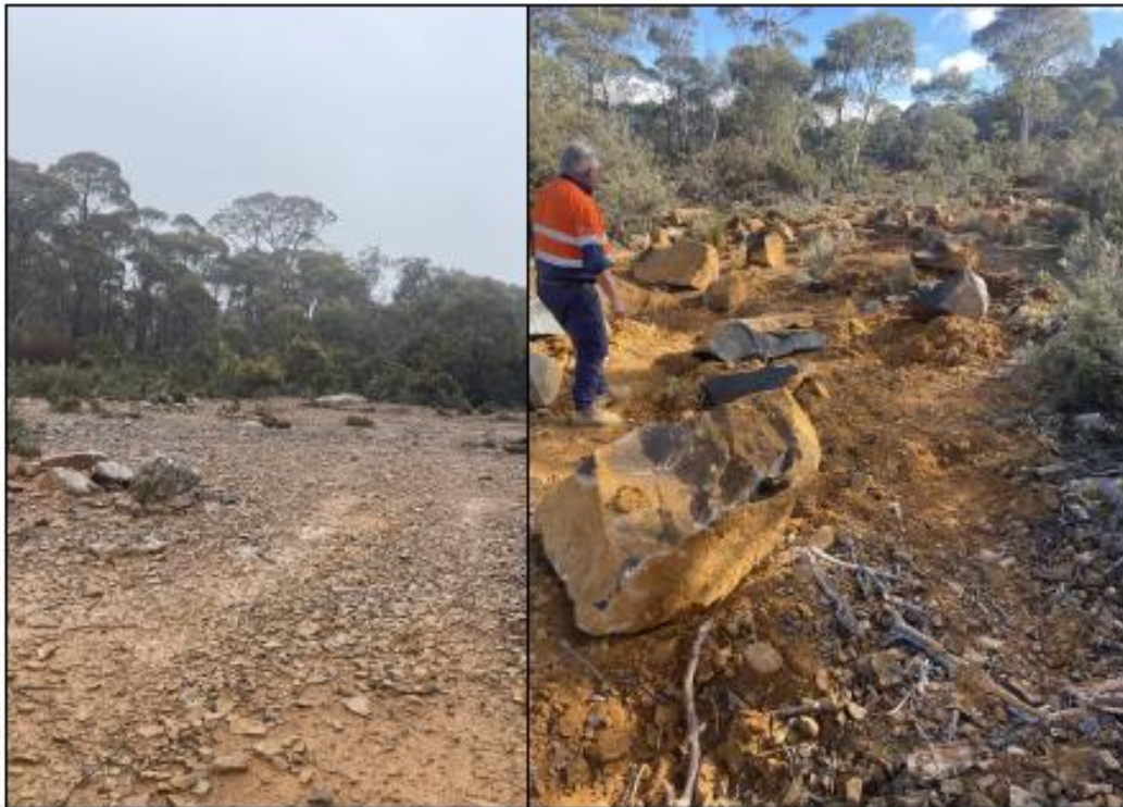
Figure 5. Left: the site being used for camping before. Right: Following earthworks, with locally sourced boulders distributed throughout site to discourage campers, ready to be planted out and brush matted this week.
